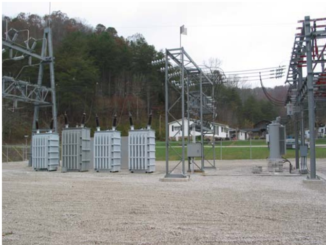
Transformer station near residential house before
