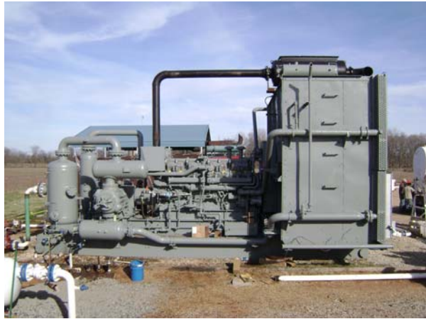
Natural Gas Compressor
